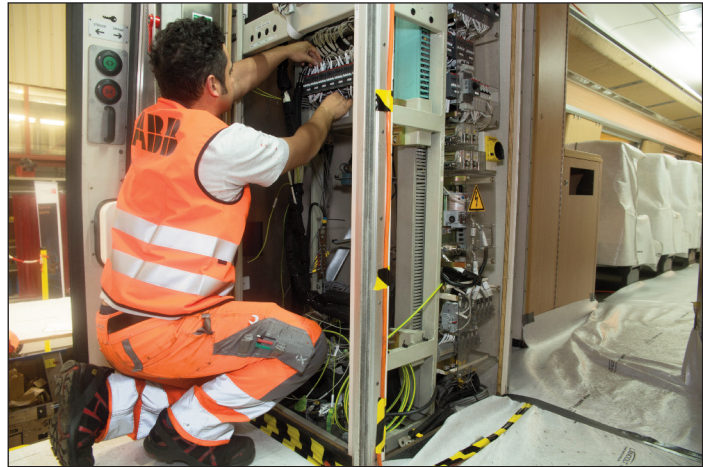
Installation of new systems in an old design configuration, and refurbishing some of the original components, is time-consuming work.
